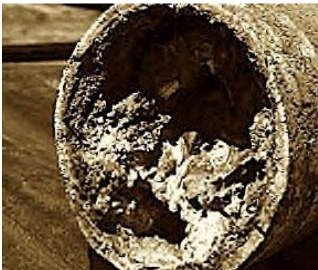
A picture of what can happen when FOG gets into the sanitary sewer system and the problems it creates.
