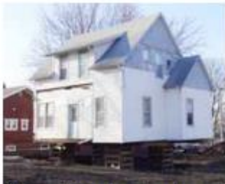
This residence is undergoing a foundation and porch alteration. A project of this degree requires thorough review.
